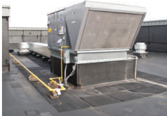
One of Princeton Windrows' high efficiency rooftop HVAC units
