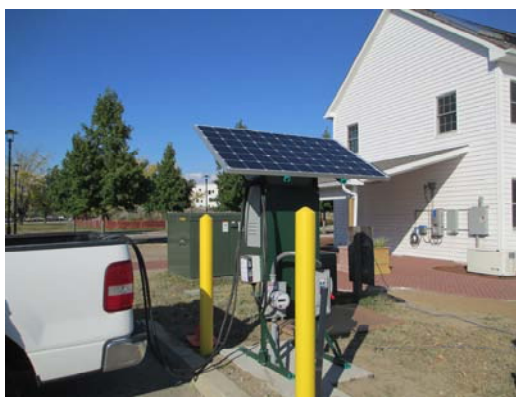
EVPV installed next to net zero energy GridSTAR house at Philadelphia Navy Yard.
